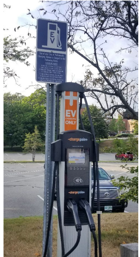
Electric Vehicle Charging Station at City Hall
